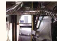
GAS OR OIL FURNACE
